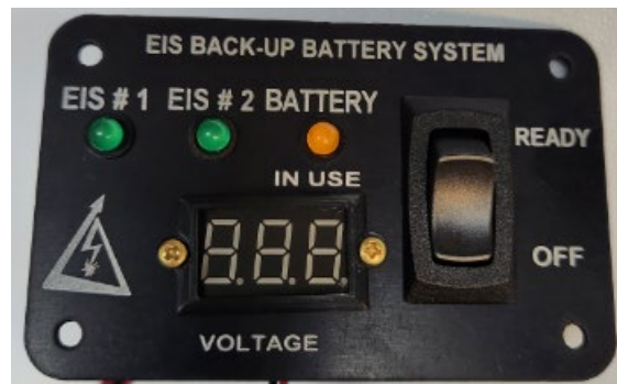
Figure 1: EIS Back-up Battery System Panel
